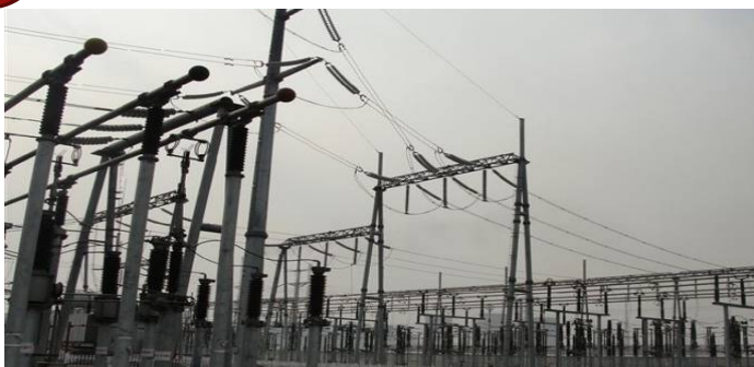
Captive power grid
